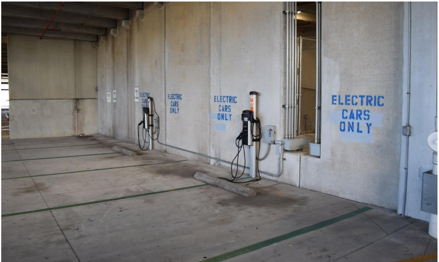
“Level 2 Charging Equipment in Pierce Street Garage. Photo Credit: Hillsborough TPO”
