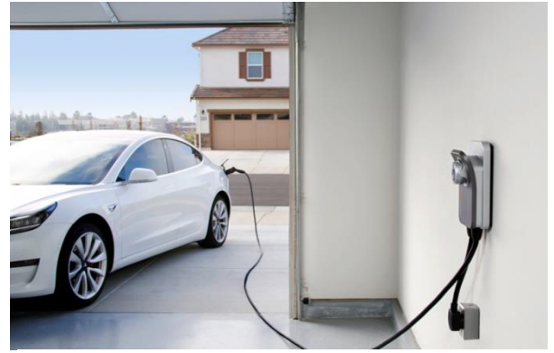
"Typical At-Home EV Charging"
