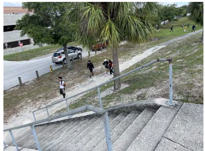
Image 61: Sand on Sidewalk and no ADA Ramp
