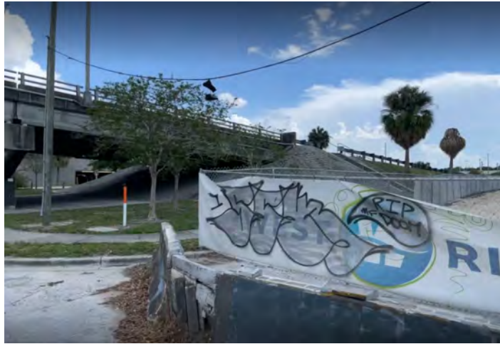
Image 67: Debris Blocking Access to Pedestrian Path
